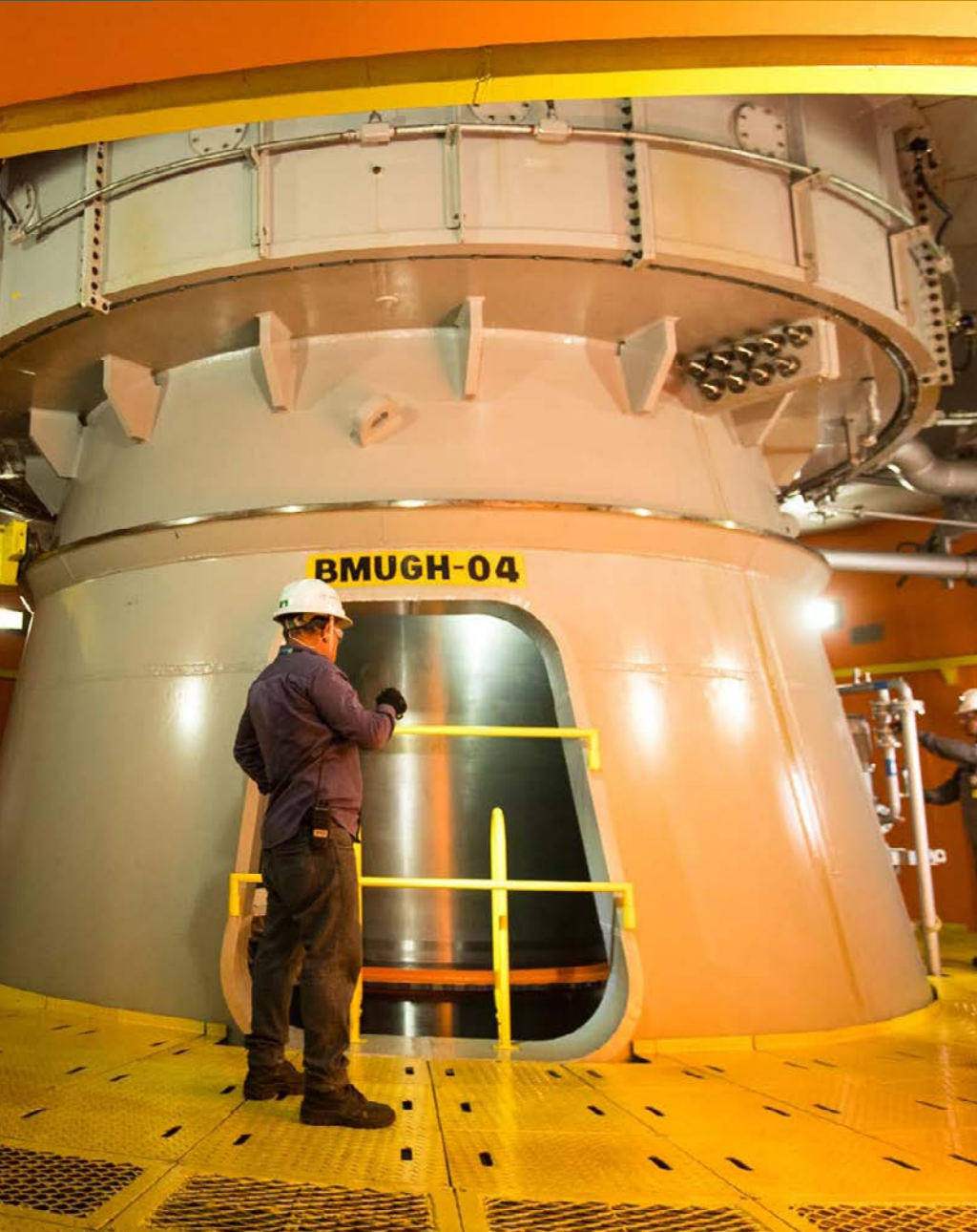
Turbine cone of Generating Unit 04 of Belo Monte HPP
