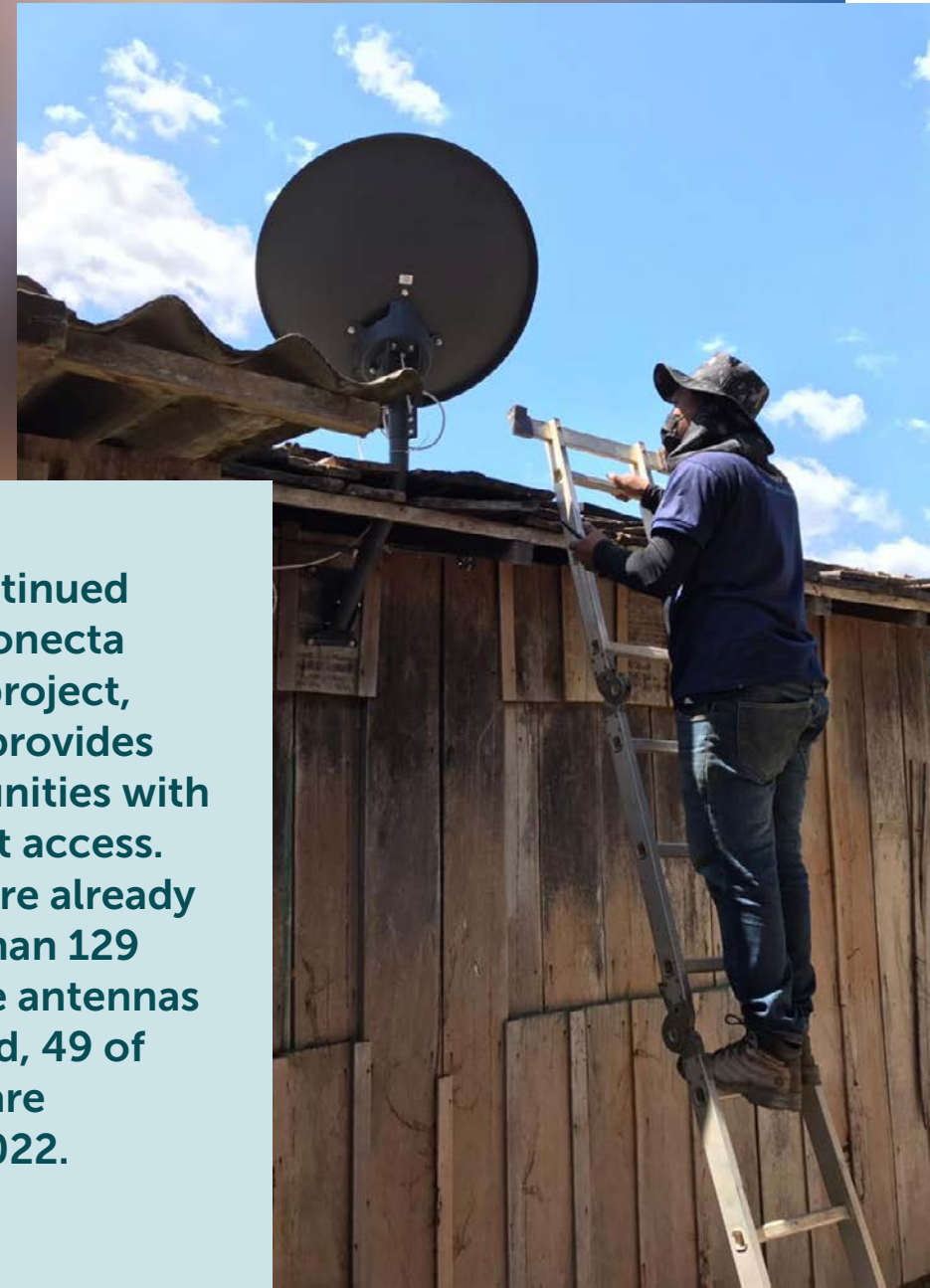
Conecta Xingu – Internet installation in the community of Volta Grande do Xingu
